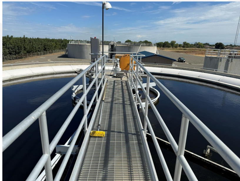
City of Live Oak's WWTP
